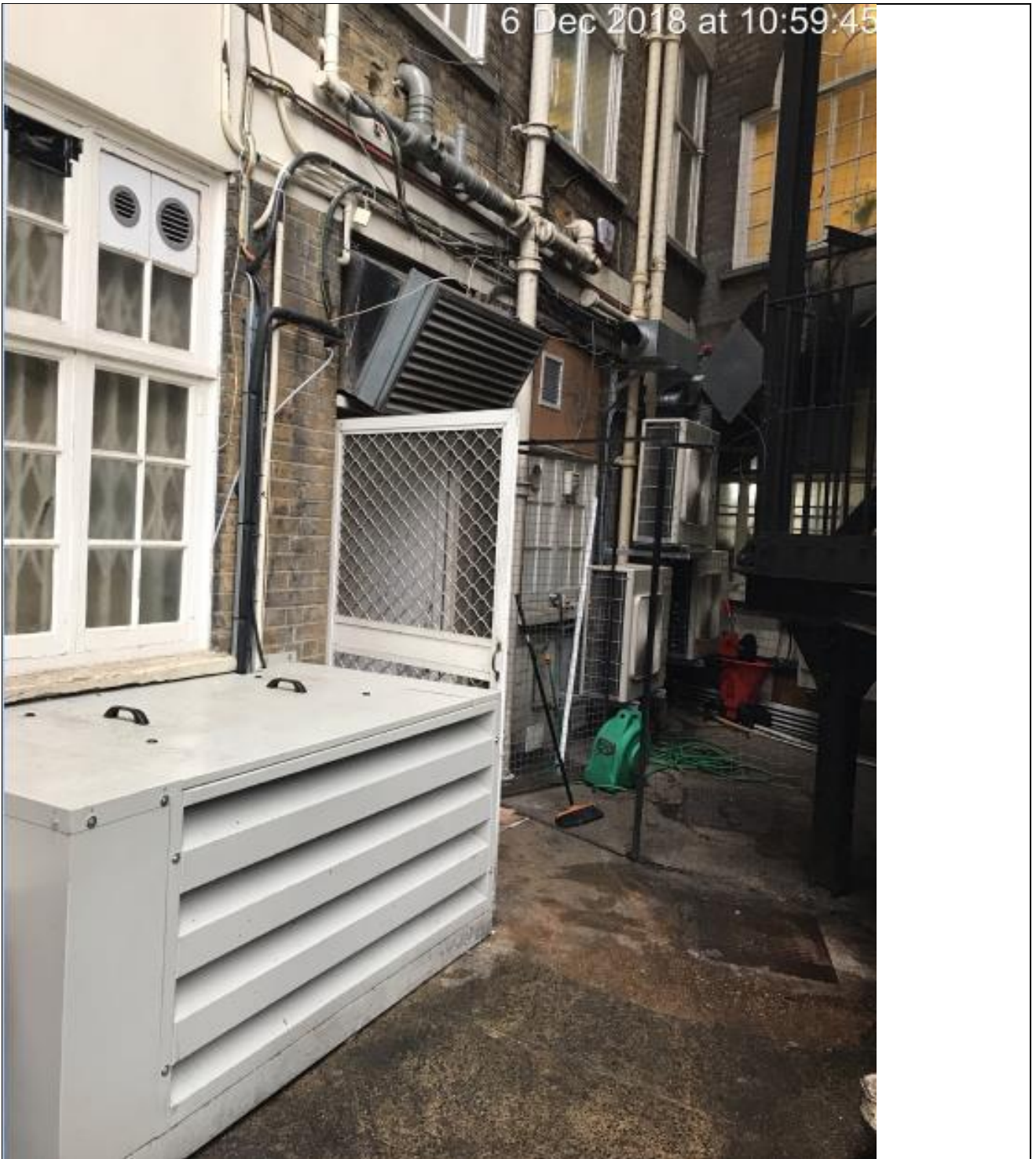
Cold room condenser – photograph taken 6 December 2018
