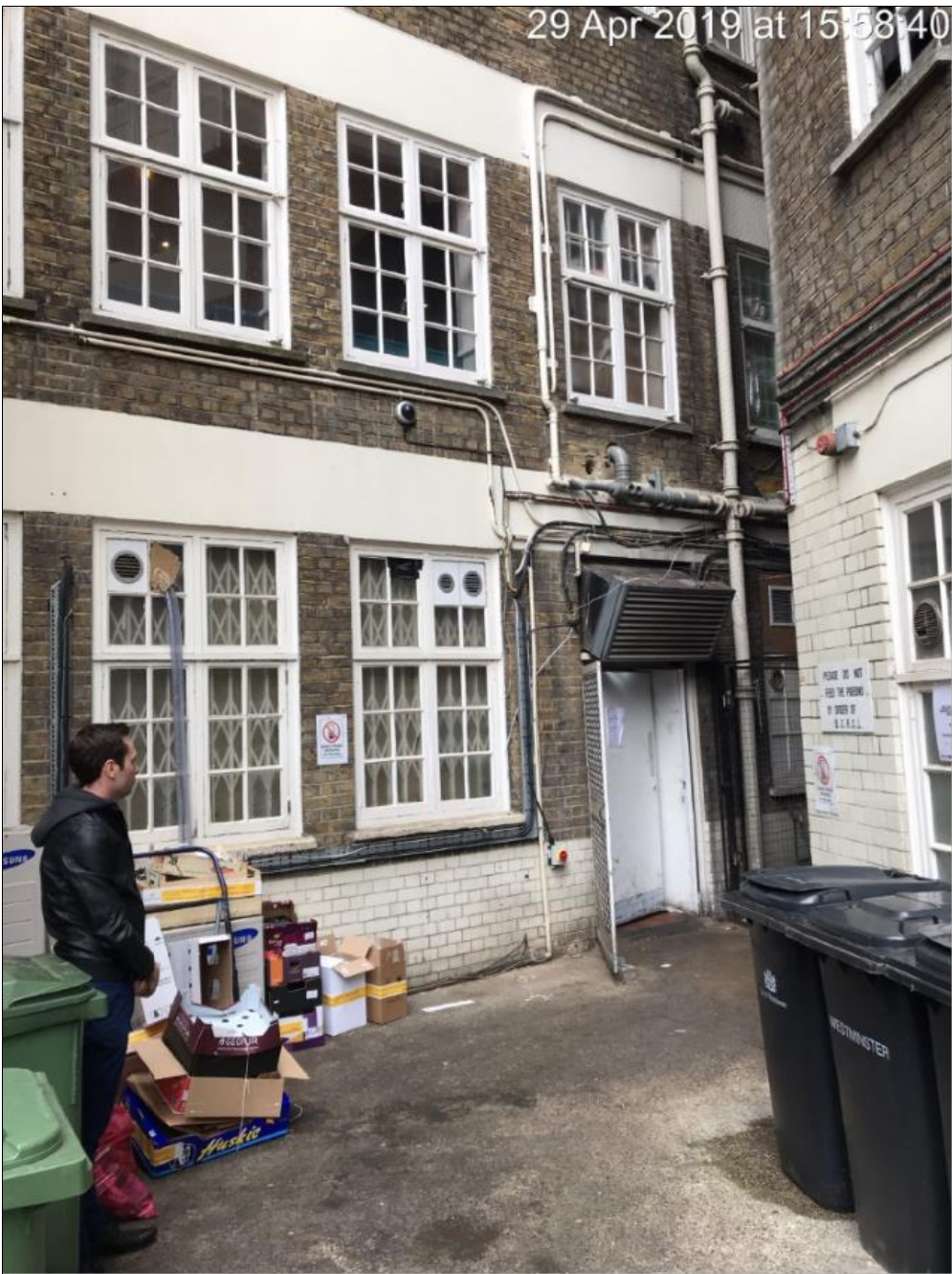
Cold room condenser removed – photograph taken 29 April 2019
